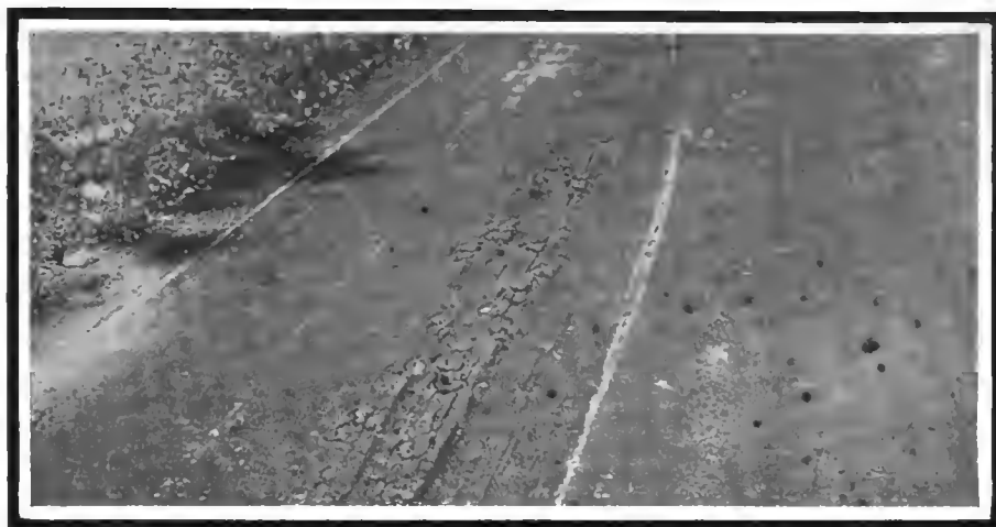
Note the effect of horse traffic on this newly repaired surface
